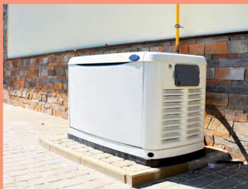
BACKUP PLAN: Standby electric generators—either portable or permanently installed, like the one pictured—can power essentials (or even entire buildings) during outages
